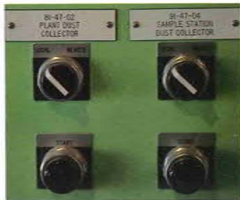
▲▼ State-of-the-art technology is employed in the plant to maintain air quality which is sampled regularly.
