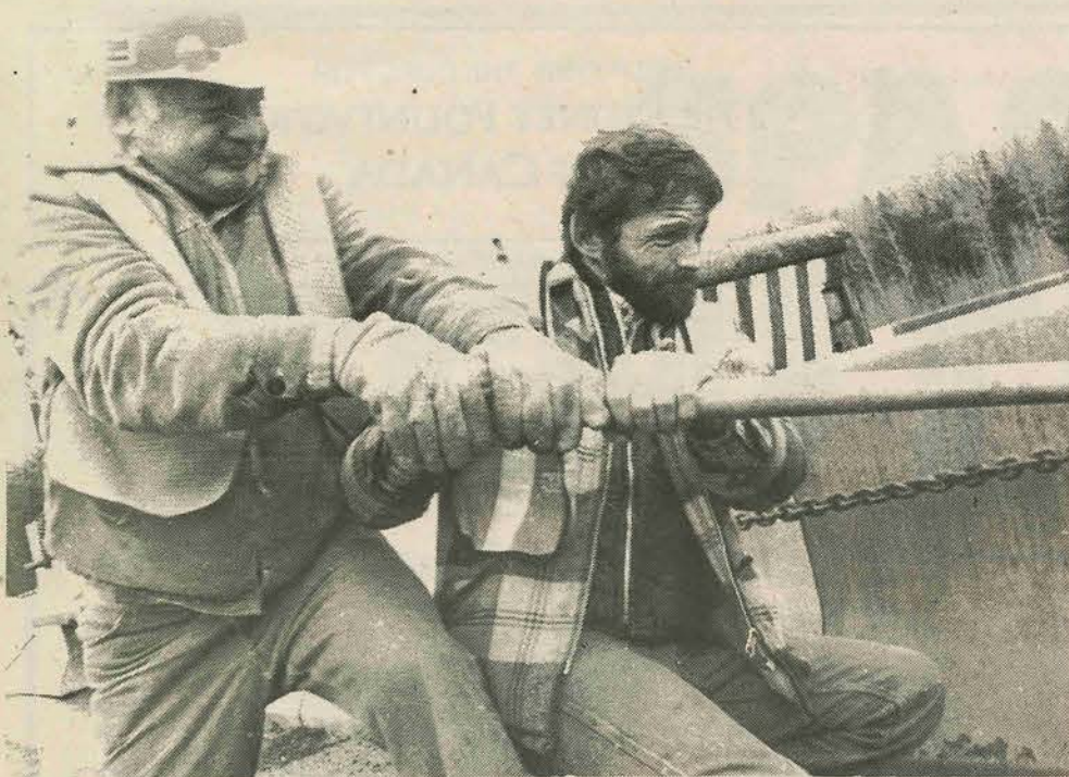
Heave-ho, me hearties! Highway work crews strain to shift one of the heavy concrete highway guards into place on the new by-pass in Sparwood.
