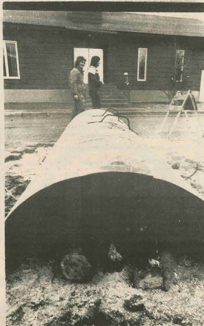
Blazing flames help to thaw out water pipes at the fountain in Centennial Square.
