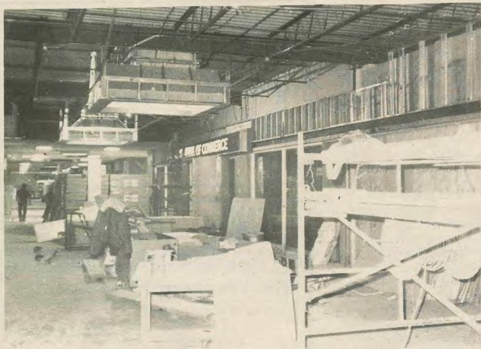
Remodelling of the inside of the Greenwood Shopping Mall is well underway, and it is hoped this phase, at the southend of the centre, will be completed about the same time as the new Overwaita store, due to open March 19.
